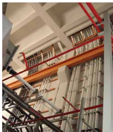
Electrical cables coated with PROMASTOP® CIS at a warehouse (below) in Ayer Rajah, Singapore.
