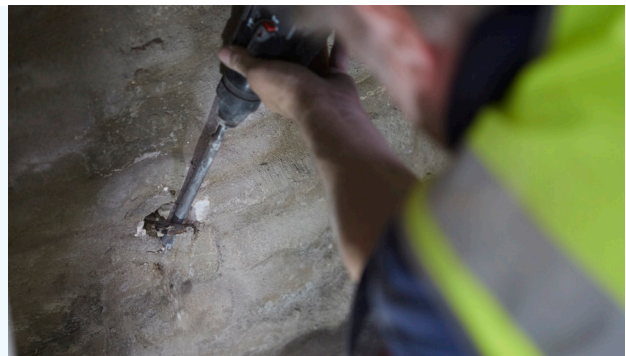
Some older properties might have hooks inside the fireplace – these should be removed.
