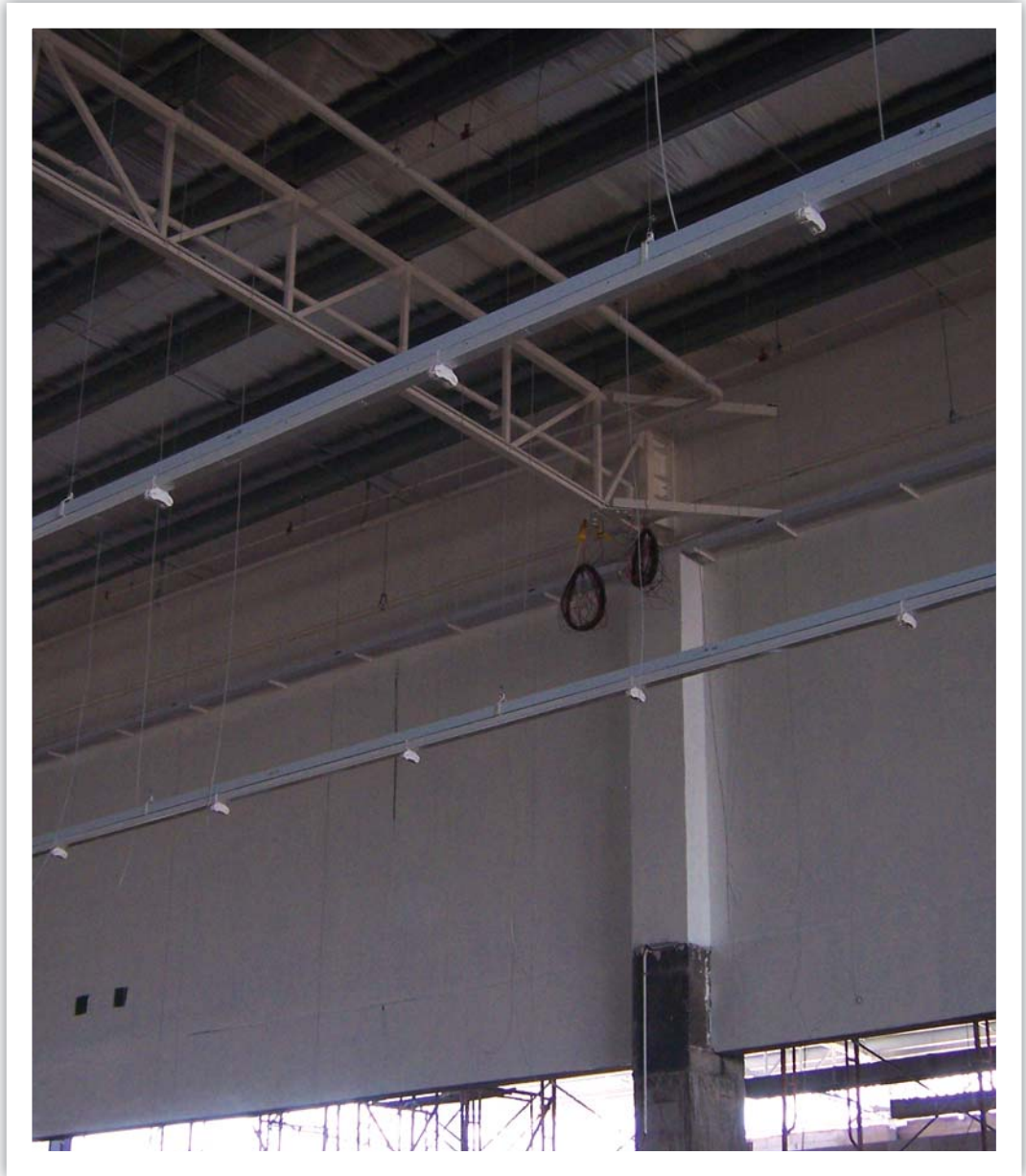
PROMINA® 60 fire resistant smoke barriers at the Carrefour warehouse in Klang, Malaysia.
