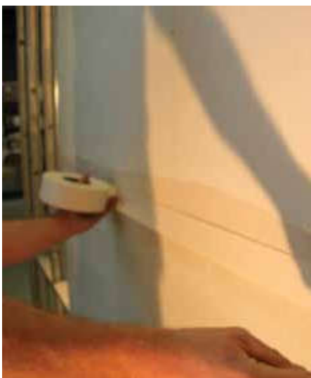
Fill joint with single, thin layer of plaster and then overlay reinforcing mesh.
