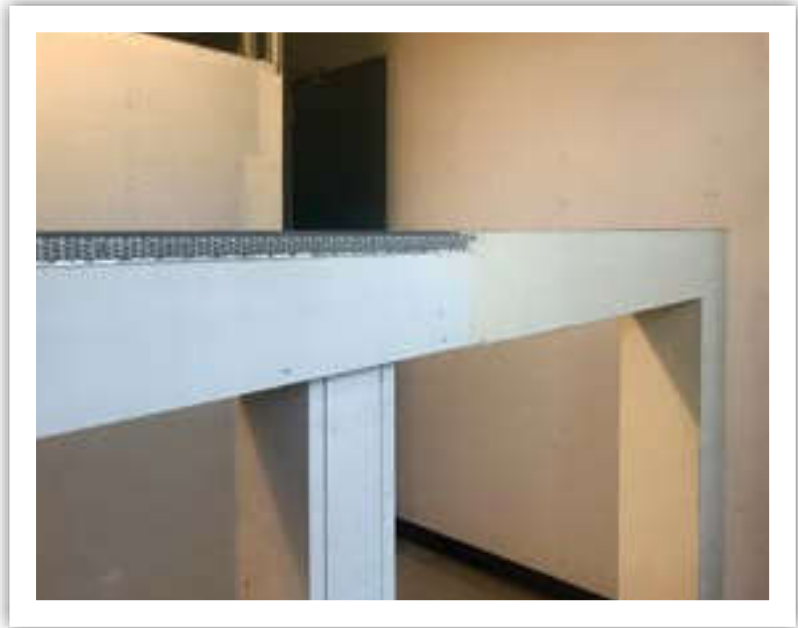
Plastering the board joints in structural steelwork and the partitions (on background of the picture).
