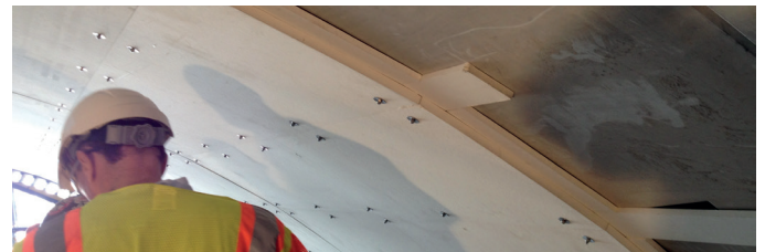
Side view of panels with leading backer strip for adjacent panel installation
